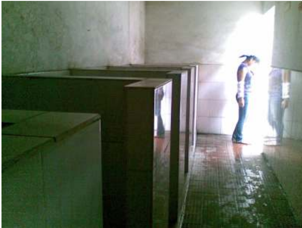
Filthy water in toilets at Yonglida.
